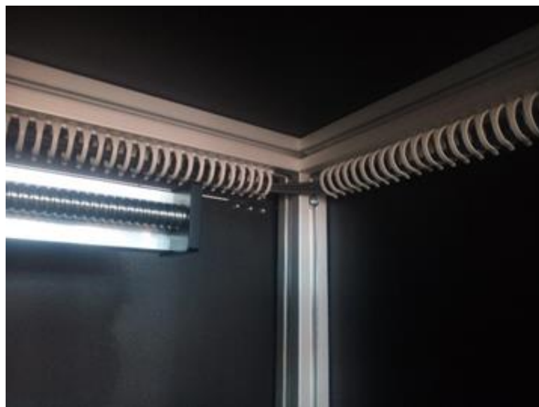
Figure 31 - Technical guides or channels to hold cablings
